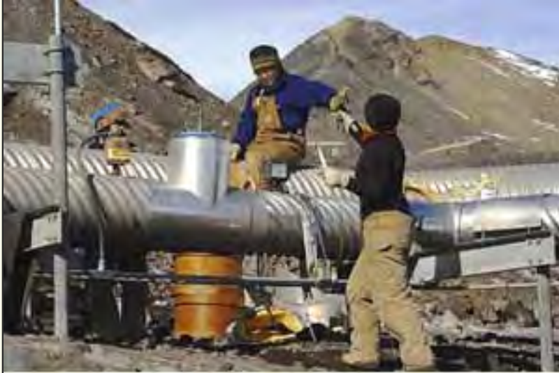
Waste Water Pipes
