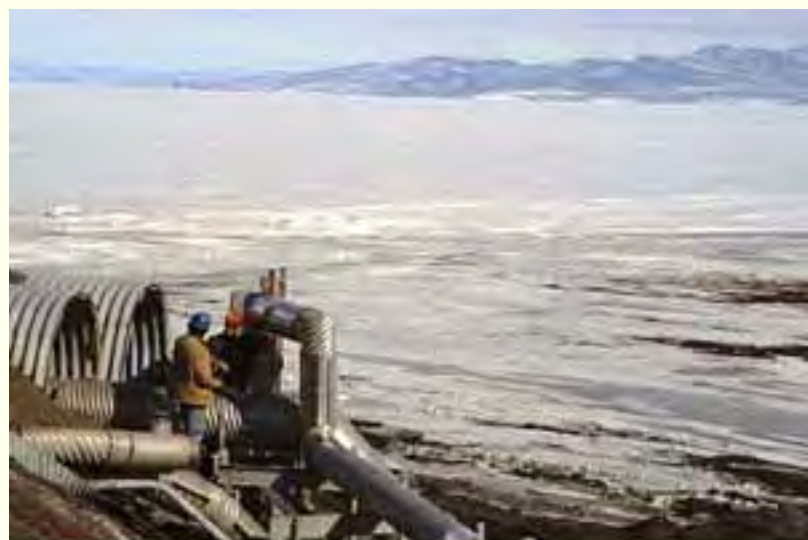
Waste Water Plumbing
